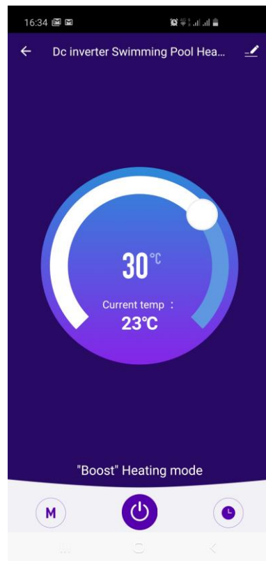
Heat pump is connected
